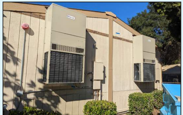
These AC units help filter all the air in the shelter, keeping our cats snuffle-free.
