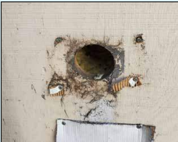
Unused exhaust ducts such as this in our infirmary are currently being addressed in our shelter makeover.
