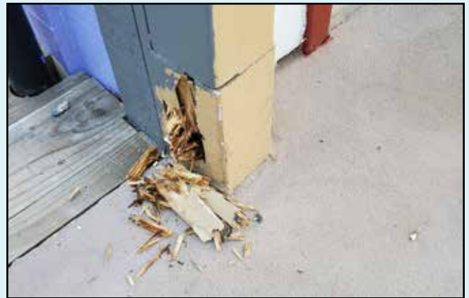
Dry rot slowly weakens the structural integrity of a building, making it a priority for ASAP to fix.
