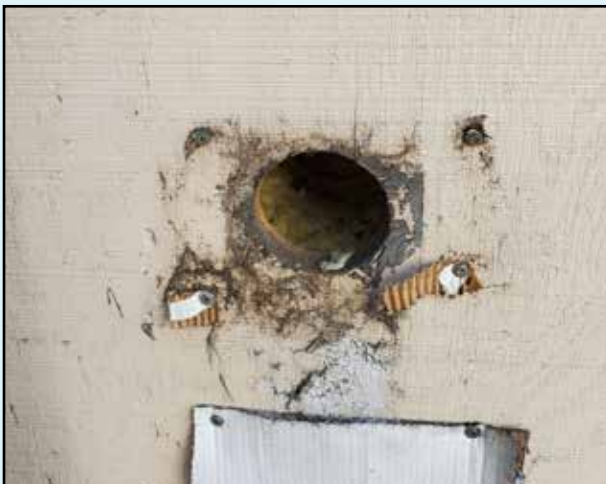
Unused exhaust ducts such as this in our infirmary are currently being addressed in our shelter makeover.
