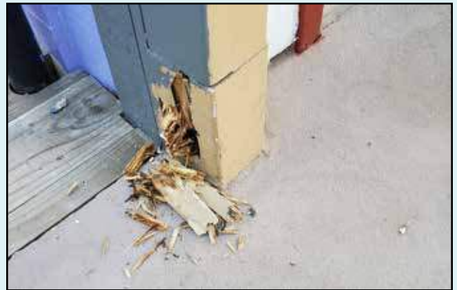
Dry rot slowly weakens the structural integrity of a building, making it a priority for ASAP to fix.
